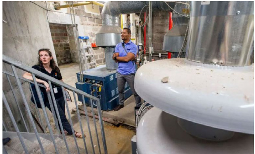
A TCHC building undergoes a green retrofit (photo credit: Toronto Star, June 30, 2022)
