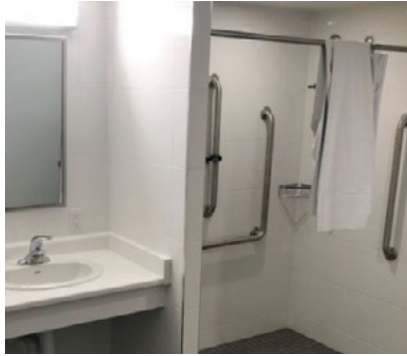
Before and after photos of an accessible washroom modification. Before: step in shower; After: accessible roll-in shower
