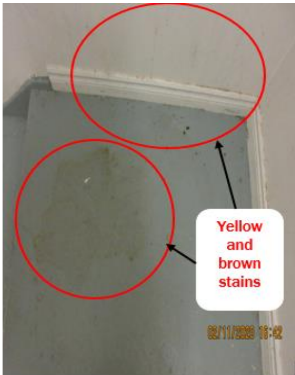
Photograph 1: Staircase not properly cleaned
