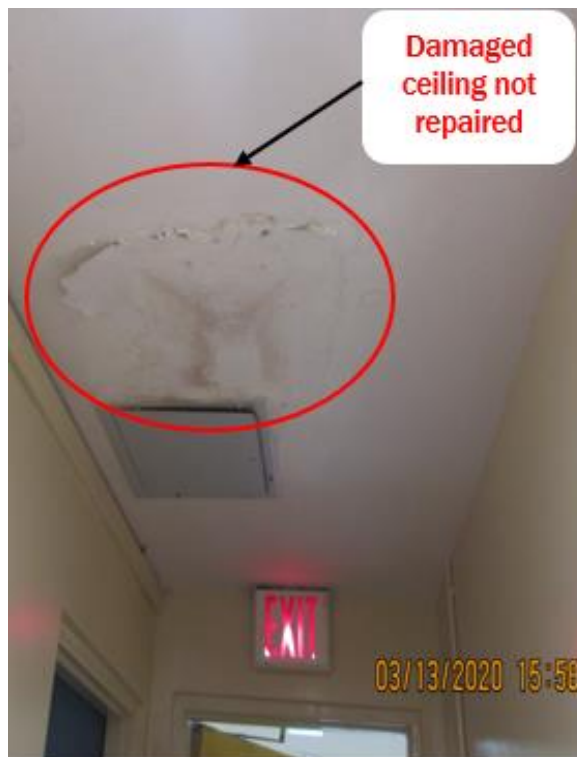
Photograph 6: Damaged hallway ceiling was not repaired
