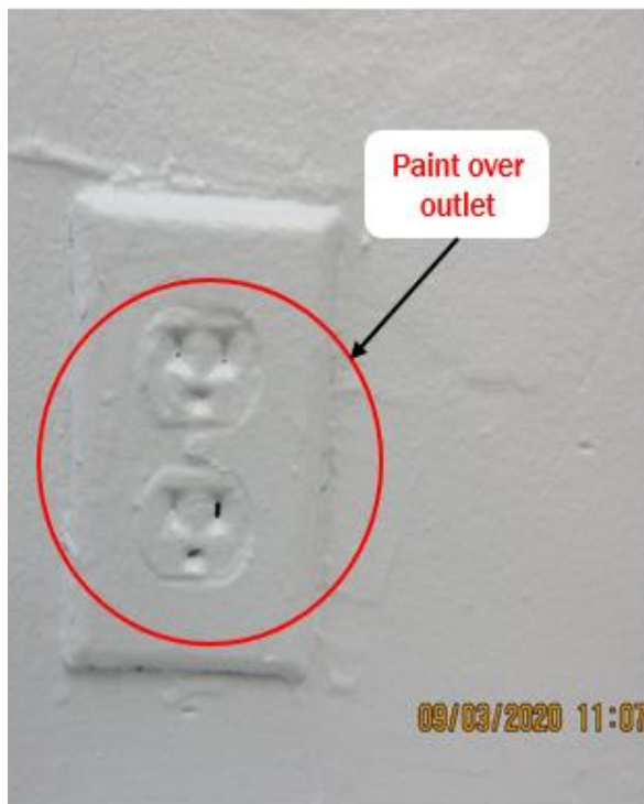
Photograph 2: Paint over electrical outlet at vacant unit
